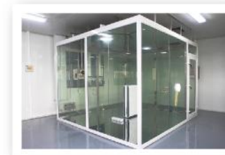
30m 3 Test Room
